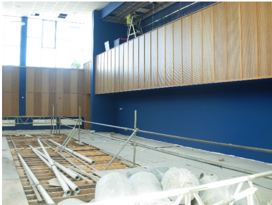
New Technical Gallery (top) with alcove underneath into which the retractable bleacher seating will fit. New solid oak to be installed and 'sprung floor' strengthened
