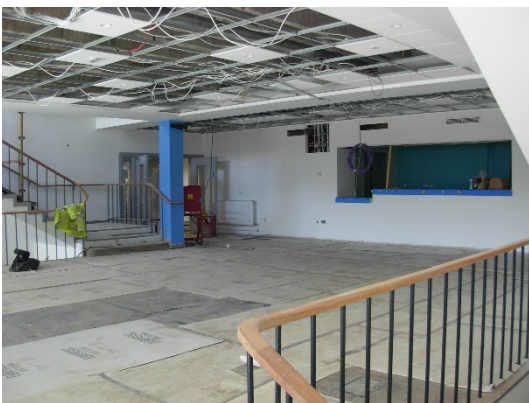
First floor bar and circulation area – original parquet flooring is being retained and
