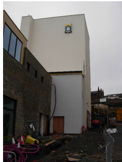
Northern elevation – fly-tower repointed and painted, new build sections (bottom left) and groundworks in preparation for new loading bay
