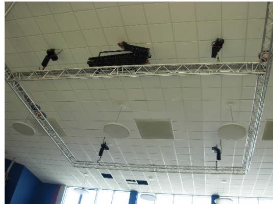
New ceiling, general lighting and fresh air vents. New figure-of-eight lighting rig suspended from 6 electric winches for ease of operation/maintenance.
