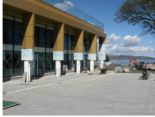
Southern elevation – new two storey glazed curtain wall and roof terrace, new clad columns (bottom two sections of cladding will be installed following completion of paving); new hard landscaping
