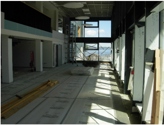
Ground floor café area, with views out to the Clyde and the Castle Gardens
